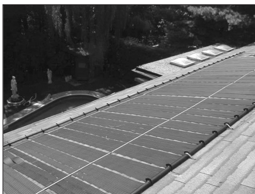
solar pool heater
